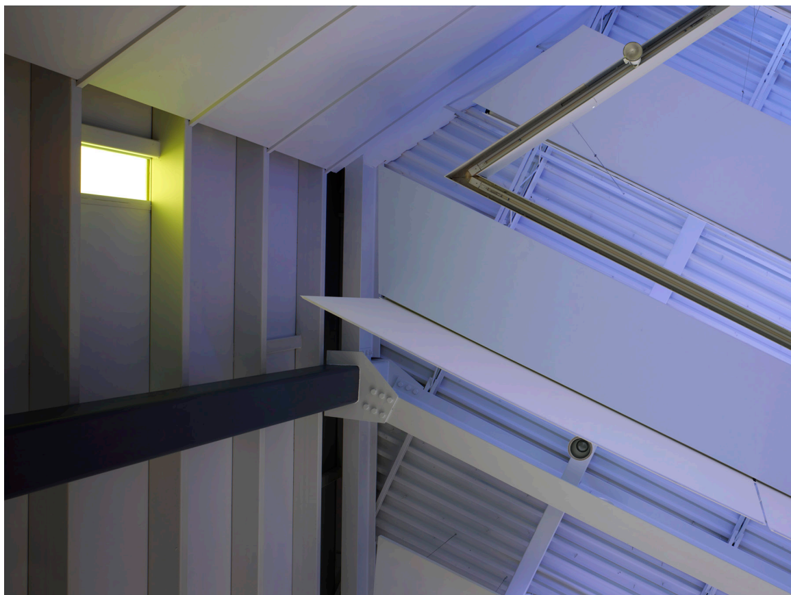
A ceiling detail in the Performance space shows the acoustical panels and tunable fabric banners as well as the light bar.
