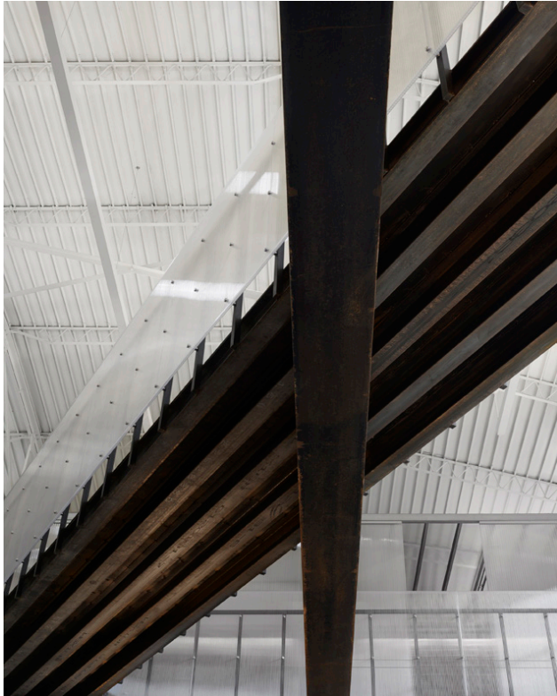
View from below of the new steel bridge and historic wide flange beam. We left the steel exposed and waxed it to keep it from rusting. The 1930s bowstring truss ceiling and deck is visible.
