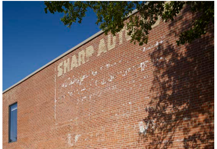
Partial west elevation showing the original ghost sign still in place. New windows were added on the east and west which were surfaces that were once adjacent buildings.
