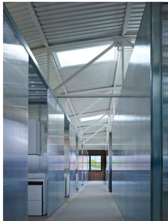
Second floor gallery corridor illustrating the 1930 bowstring truss structure and deck. The polycarbonate wall finish appears to be visually "liquid." There is reflection, transparency and shared light.
