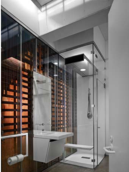
In the spirit of exposing the construction components inside walls, we chose to expose all of the refrigerant lines for the mechanical systems behind glass in the ground floor toilet. Note the duct penetrates the shower enclosure both for air delivery and lighting. The custom ADA handrail/toilet paperholder illustrates the quality of detail throughout the project.
