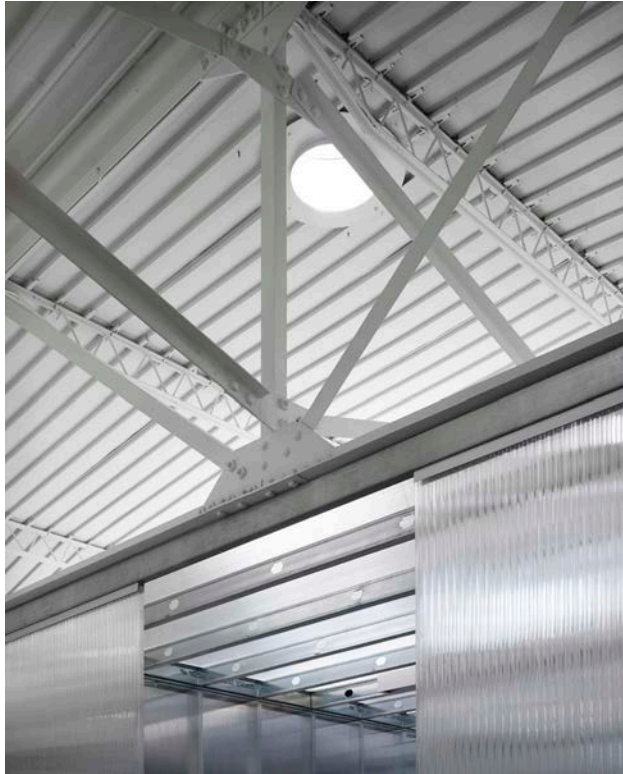
Bowstring truss deck and detail showing the Solatube skylight, metal stud office framing and polycarbonate walls.
