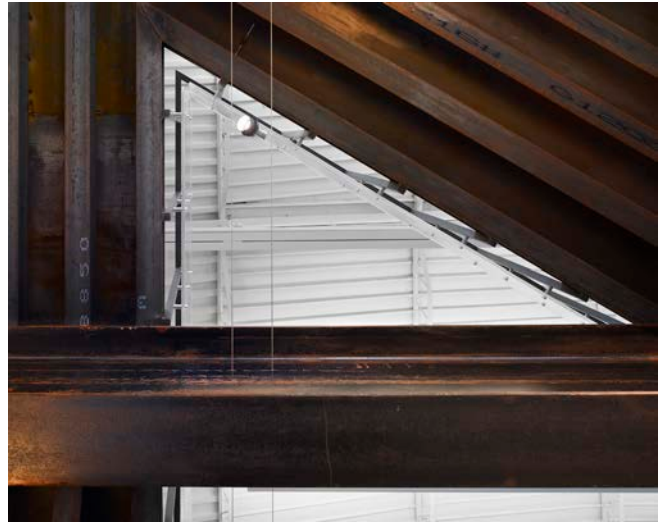
View looking up showing the historic steel beam supporting the new steel bridge. The view exposes the original barrel vault ceiling.
